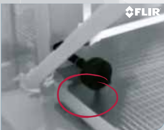
A leaking pressure gauge.
